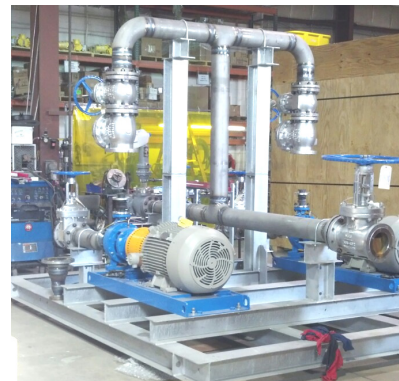
Pumping System for delivering fluid to spray nozzles
