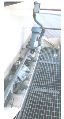
Header with Spray Nozzles at
