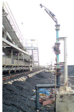
Spray cannons and stanchions for stockpiles
